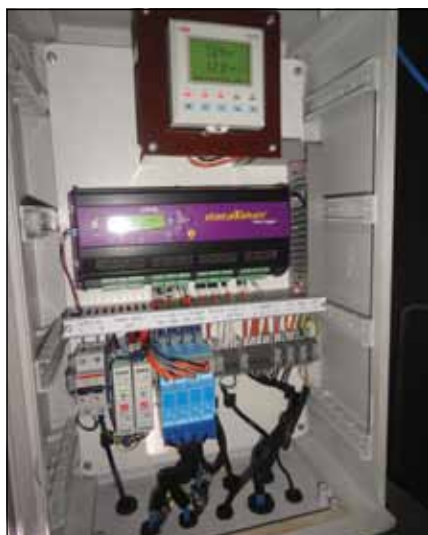
The monitoring system collects data from hydrogen sensors, a CD plate, pH probe, dissolved oxygen probe, and current input monitor to confirm the operation of a ventilation system.
