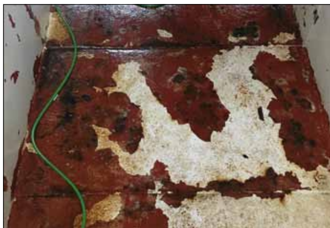
Coating delamination: automotive process plant – rinse tank.
