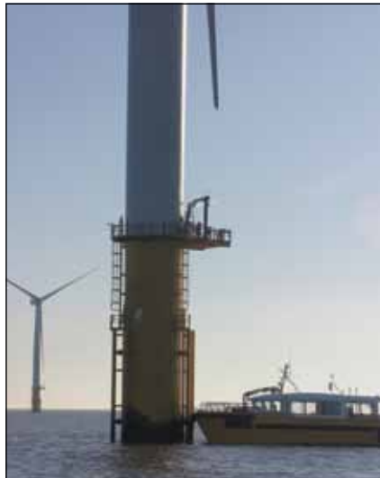
A crew prepares to offload anodes for a cathodic protection system designed to protect the interior of the wind turbine's monopile.
