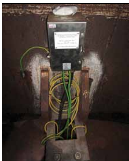
The junction box, installed above the lower platform, connects the anodes to the structure.
