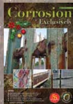
Cover: A corroded palisade fence, information sign and a security enhanced gate in aggressive coastal conditions.
