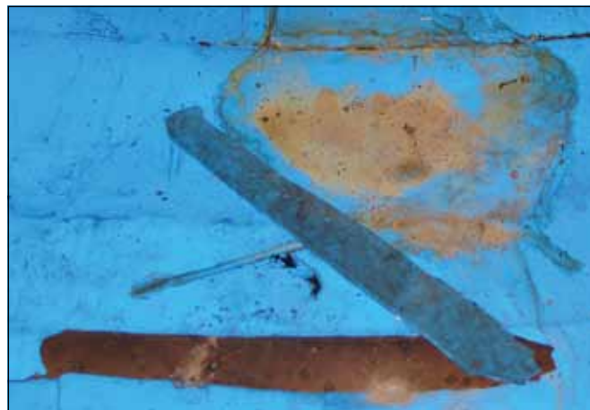
Coating delamination, blistering and cracking: flooded field joint adjacent to scour valve.
