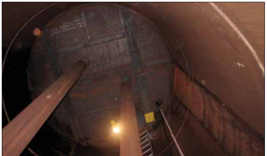
The sealed portion of the monopile below the lower platform.
