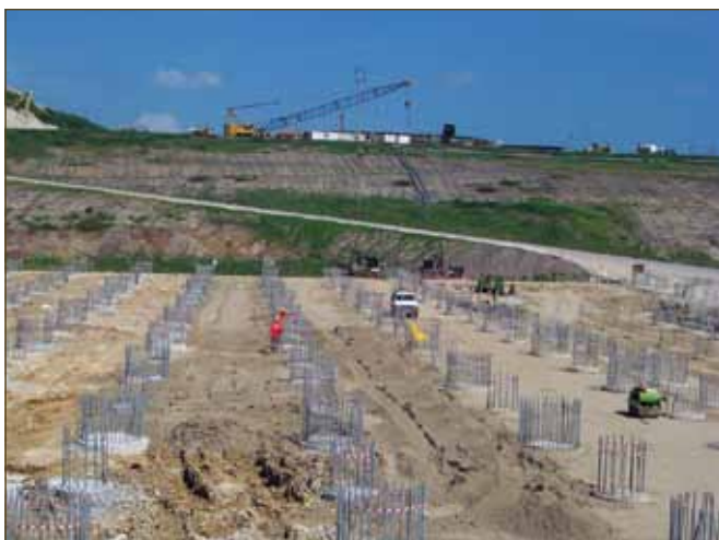
Changi treatment facility, Singapore.
