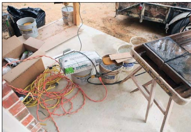
Slip or trip hazards.
