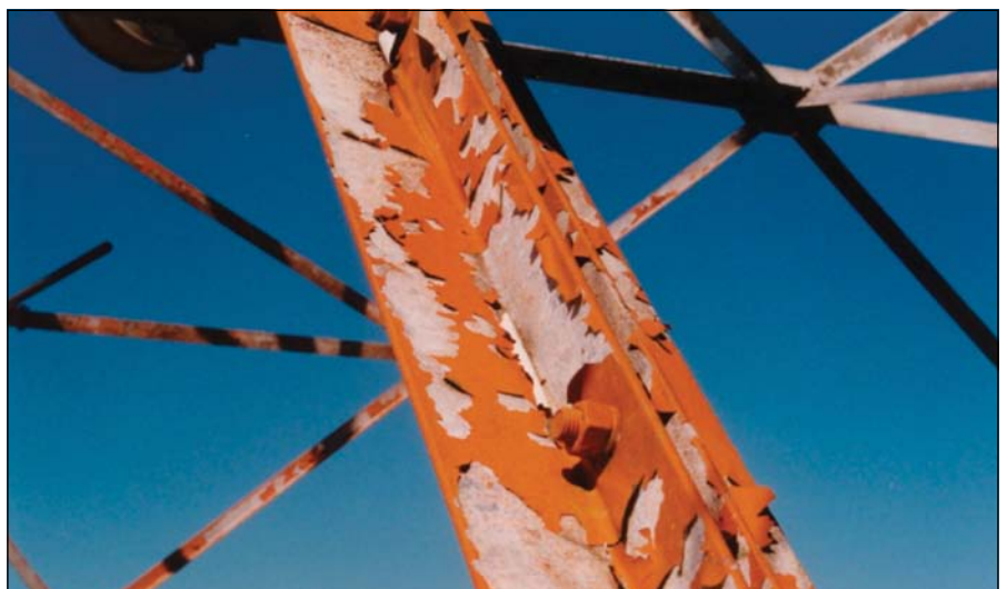
Figure 2: In some instances, the coating system will spectacularly self-detach from over the galvanizing.
