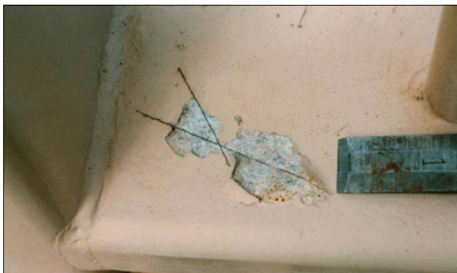
(Above) Figures 3 and 4: A common finding is that the coating system is drummy with very poor adhesion, and underneath the film is a prodigious amount of white zinc corrosion products. Visible rusting of the underlying steel substrate (or the zinc/iron alloy layers) also quickly appears with its typical red/brown corrosion products.
