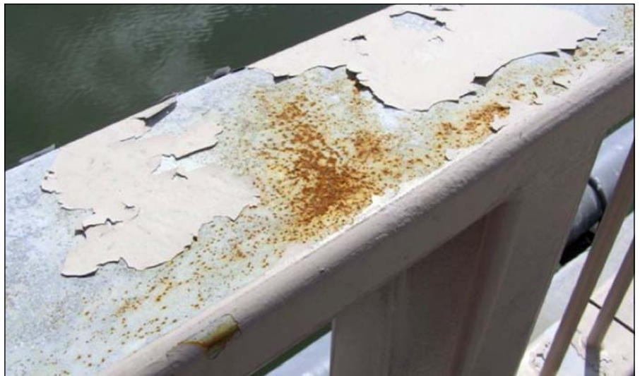
Figure 1: A typical dramatic failure of a galvanizing plus topcoat (duplex) coating system after four years of exposure.
