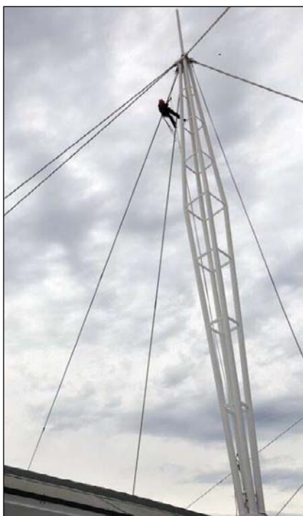
Working 20 storeys above the ground adds to the challenges of protecting structures from corrosion.
