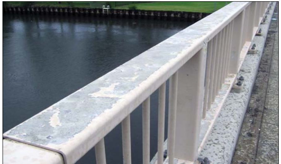
Figure 7: Often, it is the horizontal surfaces that are more affected, probably because the time-of-wetness of these is higher than on vertical members. Note the loss of topcoats on the top face of the upper and lower RHS rails, versus the uprights.
