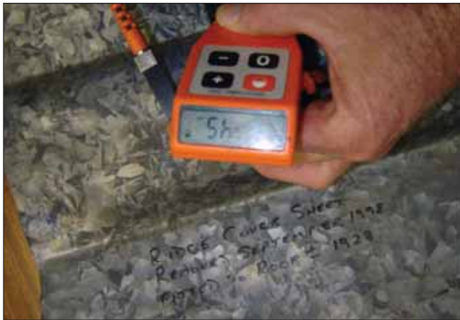
The underside of a ridge cover sheet fitted in 1928 shows a residual zinc coating of 45µm.
