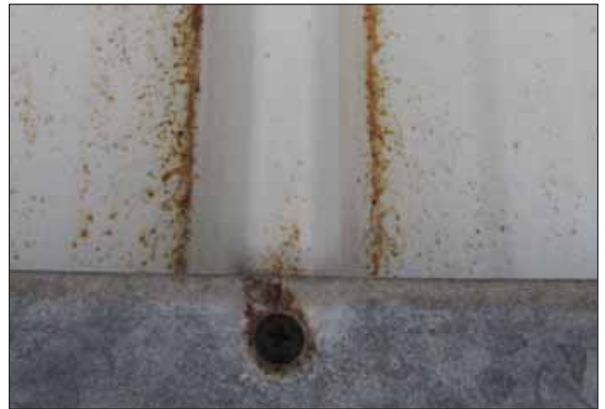
Swarf and mild steel grinding dust not removed at installation now seriously affecting roof sheeting aesthetics and ultimately corrosion resistance.
