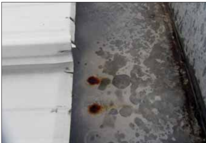
Discoloration in galvanized gutter from roof sheeting.
