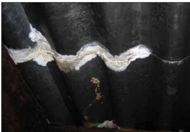
Metal corrosion at sheeting overlap.
