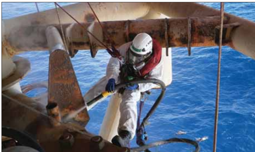
Preparing the steel of an offshore structure for priming and spray coating.
