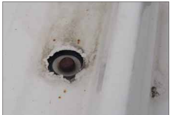
Failure of sheeting at fastener due to bi-metallic corrosion.
